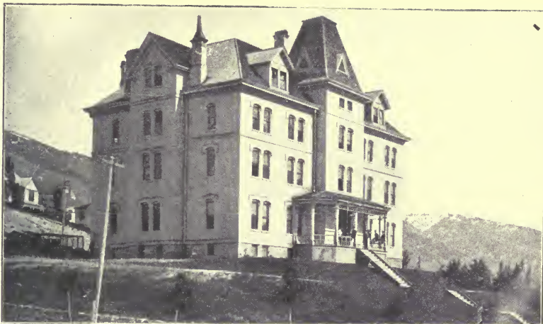
This building is being remodeled and beautified—to be used wholly for Domestic Science and Arts. It contains an elevator and all modern equipment, and will be one of the best Domestic Science and Arts buildings in the whole West.
